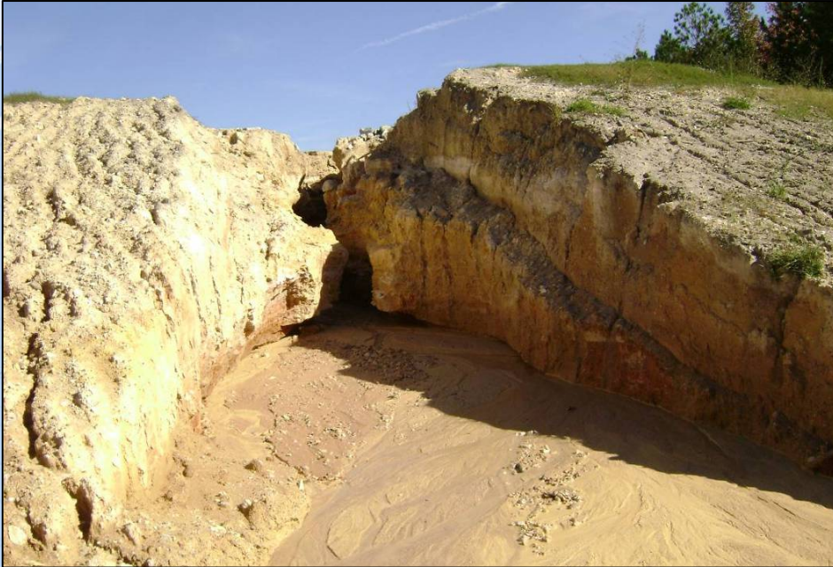
Failed Sediment & Erosion Control Structure Draining into Crane Creek
